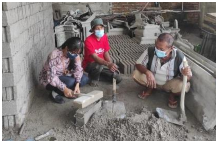
Figure 2. Implementation of direct practice of making bricks with a mixture fly ash
